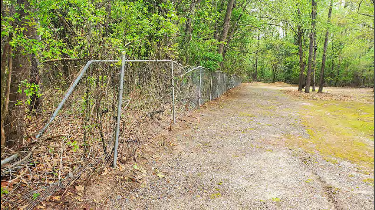
Figure 81. View of southern fence damaged by past trees falls.
