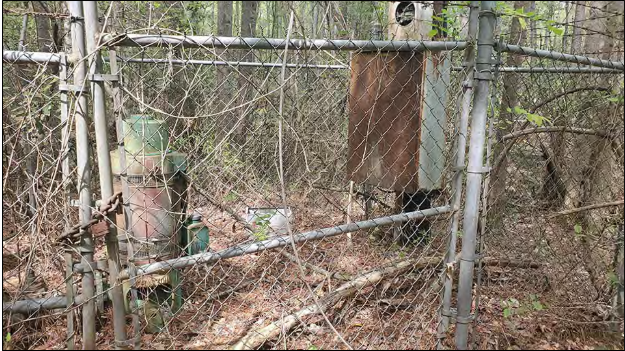
Figure 95. Abandoned pump and electrical components within area.
